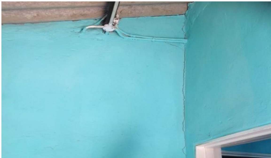
Cracked house: Auditor – December 03, 2021
